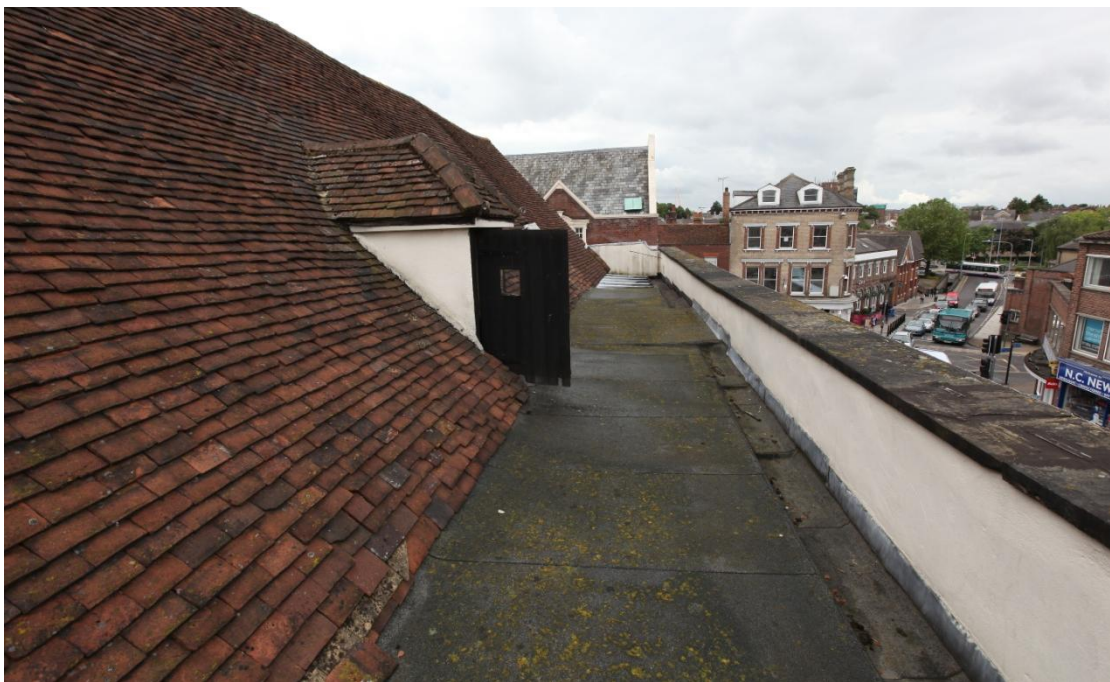
Illus. 33. The wide area of flat roof between the Head Street parapet and the tiled roof, showing the present access hatch on the left. An area of leadwork can be seen in the rear but the majority appears to be covered only in felt (possibly concealing lead). This unusual arrangement corresponds with the building’s depiction in 1745 with a low attic storey beneath a shallow roof; this was presumably achieved by adding a false vertical wall to the front of the rafters to create – in effect - a continuous dormer.
