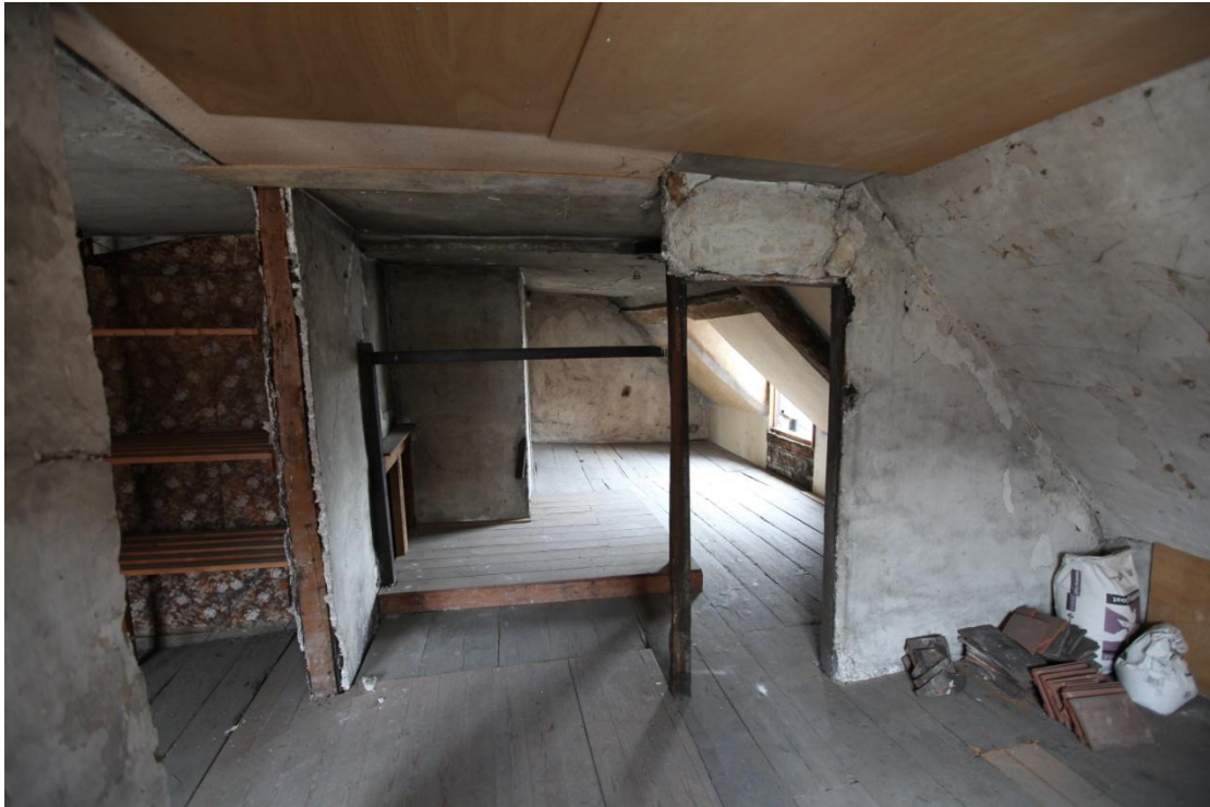
Illus. 28. The lath-and-plaster partitions in the attic of the Head Street range, seen from the north. The broken wall to the left and the patched ceiling relate to the missing chimney shown to the left in figure 17. The access to the lead roof detailed in illus. 29 below is visible in the rear to the right.
