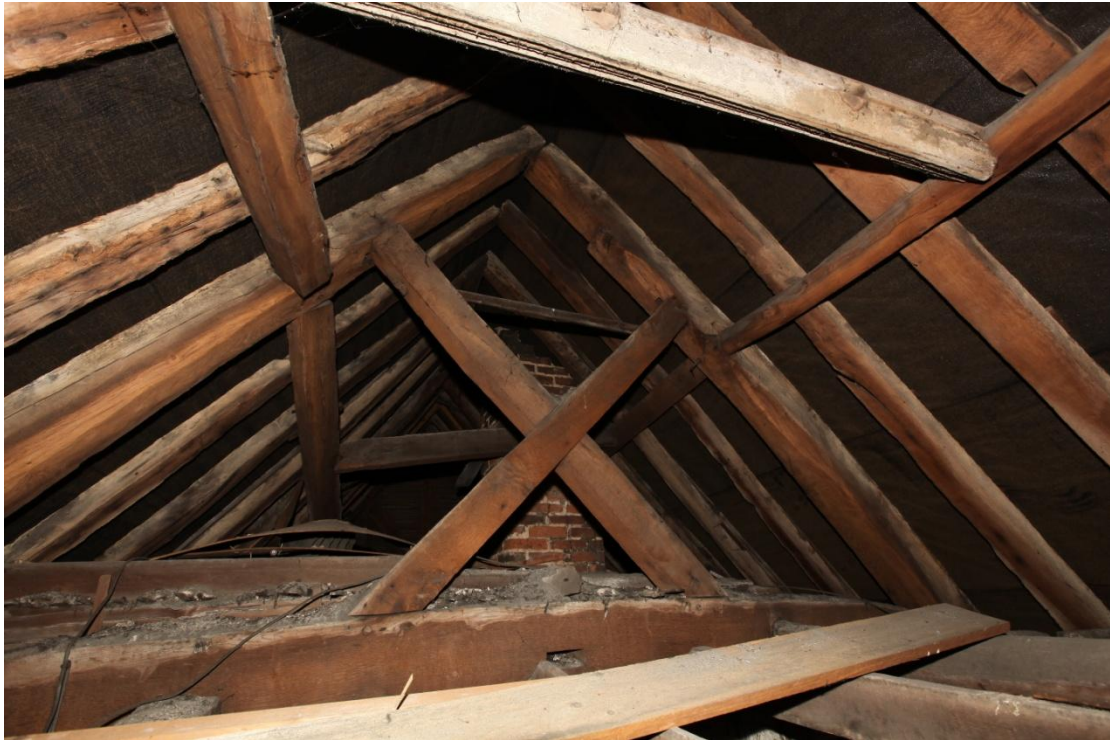
Illus. 30. The roof structure of the Head Street range, looking south towards the chimney of the main first-floor reception room which has been truncated below the ridge. The collar is Saltire-braced to the principal rafters, with two tiers of linear butt-purlins and copious re-used timber. The collar at the top of this image is a re-used early-17 th century window lintel with impressions of ovolo-moulded mullions, but may be a later insertion.
