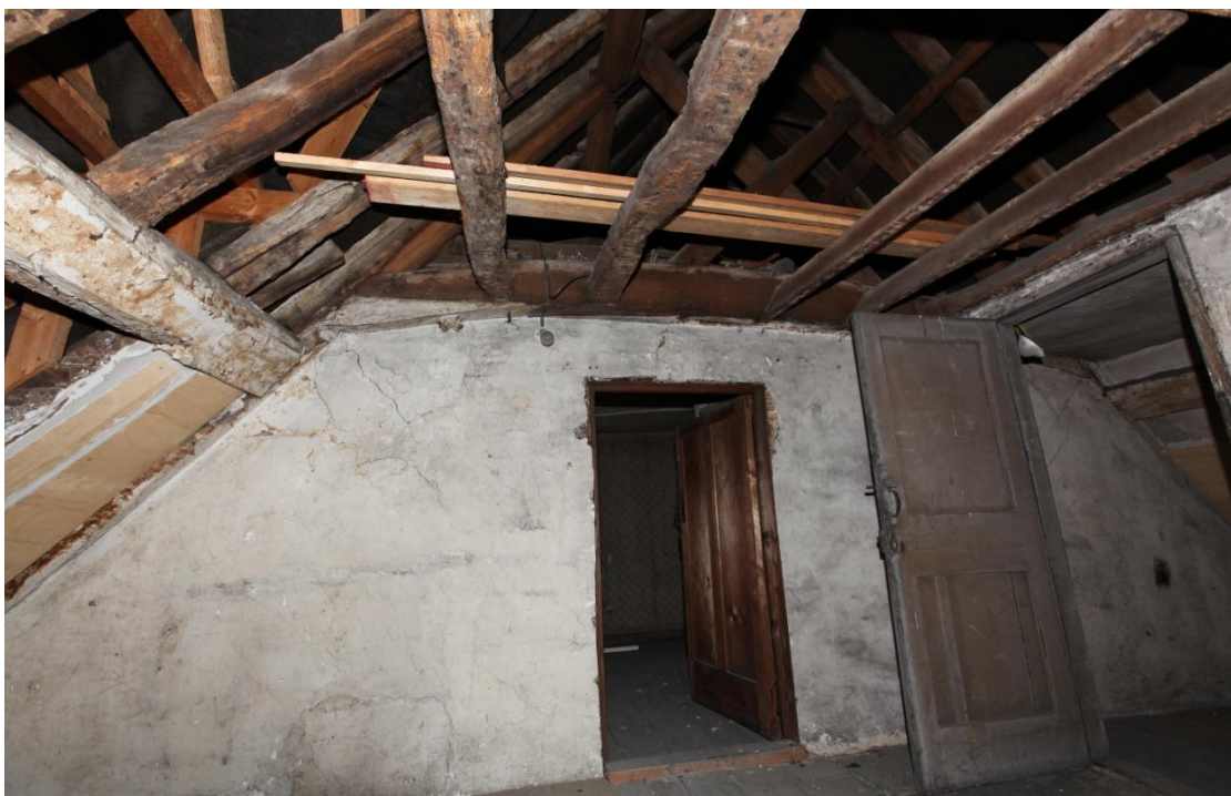
Illus. 31. The entire roof truss shown in illus. 30 above, with the lower butt-purlin to the left and the joists of a missing plaster ceiling. Most of the plasterwork in the attic appears to date only from the early 19 th century, but the collar contains a pegged central mortise that may have secured the axial joist of an original ceiling.
